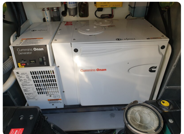
Beneteau MC5 generator
